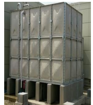
Water Storage Tank
