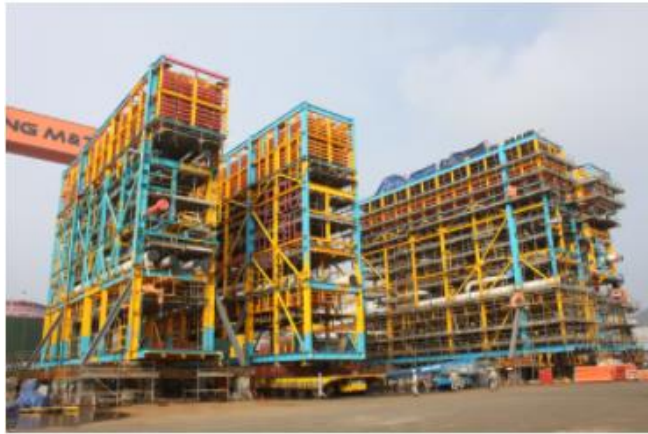
Pipe Rack Module
